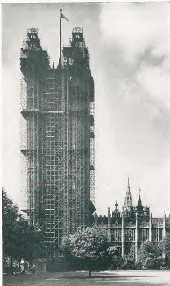
'S & L' steel scaffolding tubes in use for re-conditioning the Victoria Tower which is 75 feet square and 340 feet high.
